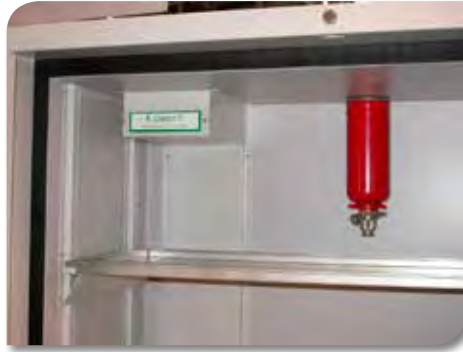
Fire-extinguisher installed in a safety cabinet
